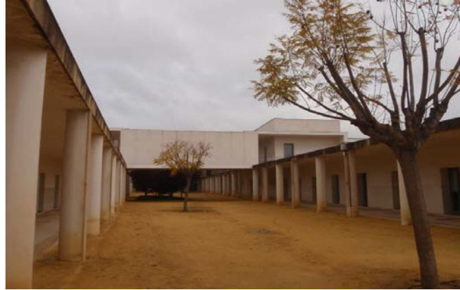
Figure 3: Place: campus, the courtyard of the Rectorate and Authorities (Rectorado y Servicios Generales) building. The aspect described: inefficient drainage and lack of waterproof or rain-resistant façade finishing. (All photos in this article were made by the author in March 2013).
