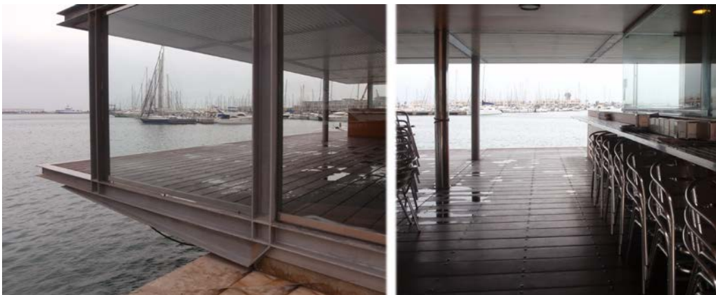
Figure 8: Place: the harbour of Alicante. The aspect described: the deck of café bar without handrails.
