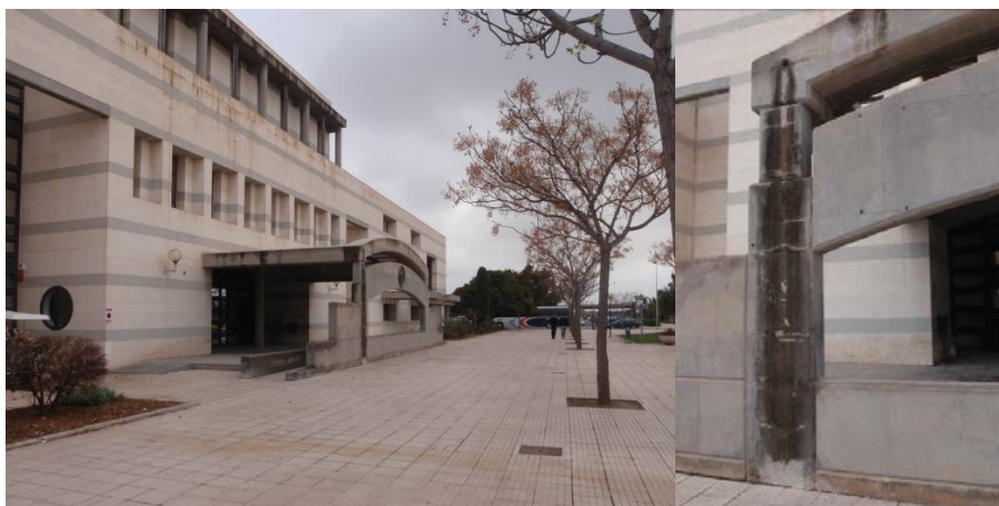
Figure 5: Place: campus, the entrance of Faculty of Economics and Business Sciences. Aspects described: decorations blocking the entrance and the lack of drainage system.
